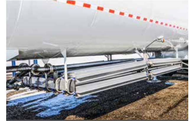
PRESSURE BUILDING COIL SYSTEM - OFF LOADING
