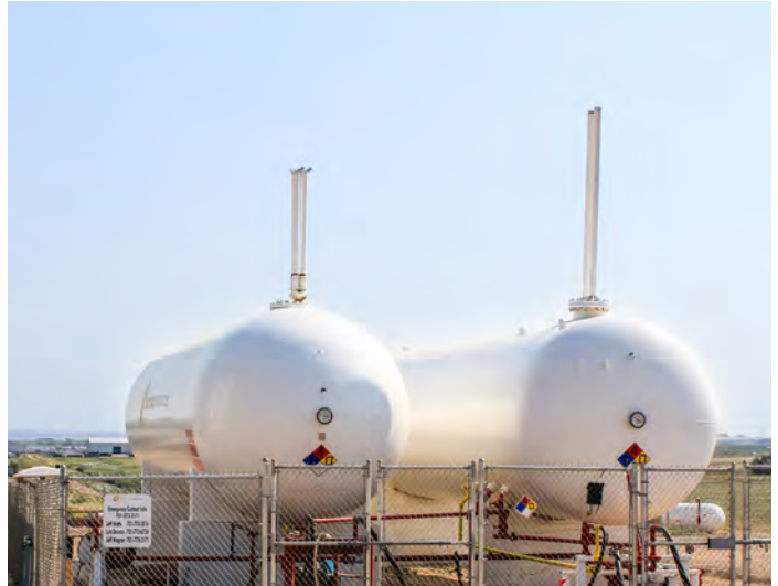
LP BULK PLANT
