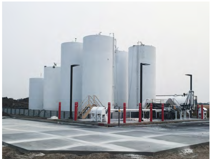
REFINED FUEL BULK PLANT
