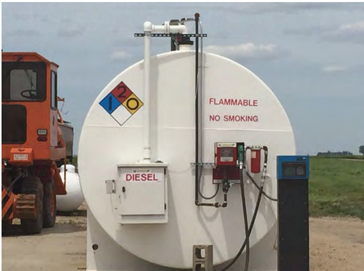
FUEL ISLAND TERMINAL
