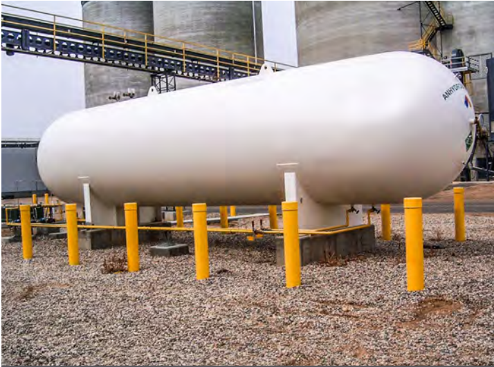
NH3 PRESSURE VESSEL
